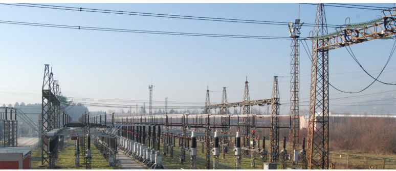
Sarajevo's substation of Elektroprijenos BiH "Copyright: CET Energy d.o.o"
