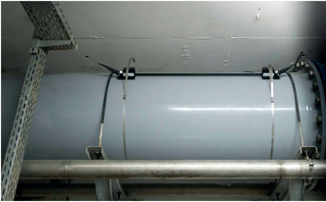
Siemens clamp-on sensors mounted on a DN800 steel pipe to measure the return activated sludge..
